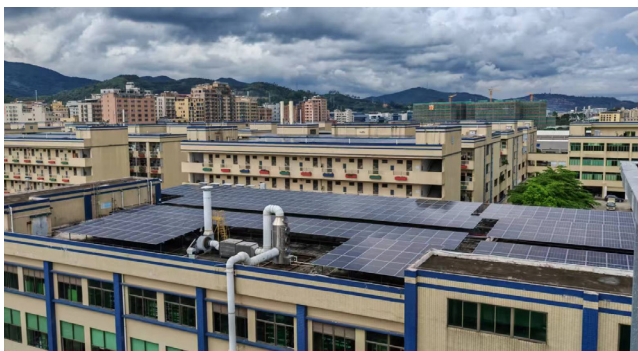
Solar panels installed at manufacturing plants
